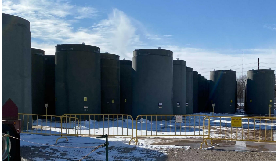
Dry casks at Dresden Generating Station, Morris, IL
